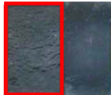
Cracking of bending section cover
