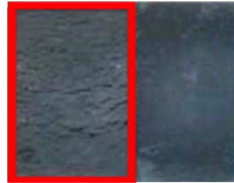
Cracking of bending section cover
