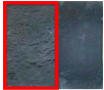
Cracking of bending section cover
